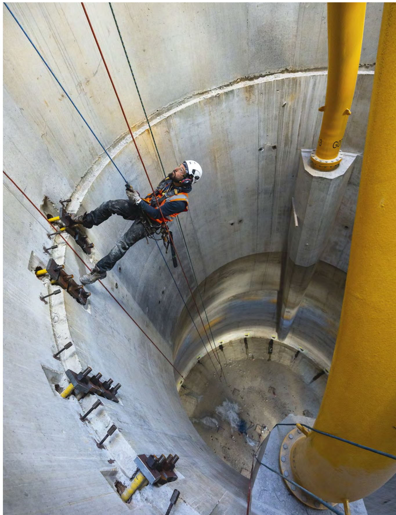
Construction of gravity-based foundations for an offshore wind farm, Le Havre, France © 2022 Petzl Distribution - Vuedici.org - Ouest Acro - Bouygues travaux publics - Fécamp offshore wind farm
