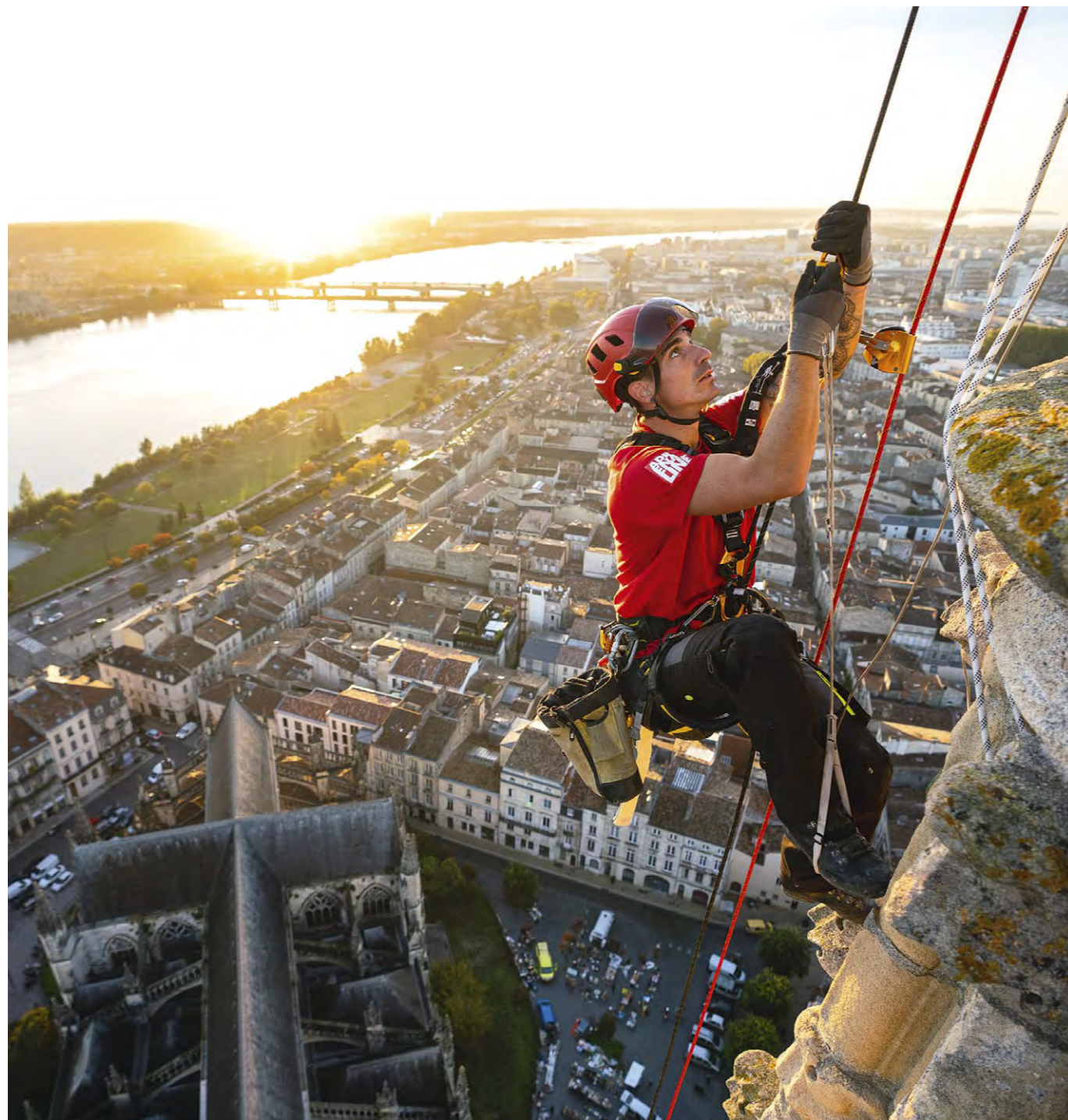
Installing monitors on the spire of the St Michel Church, Bordeaux, France © 2021 Petzl Distribution - Vuedici.org - Adrenaline - Bordeaux City Hall
